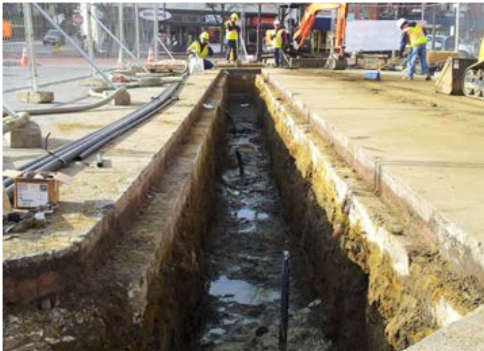
Gannett Fleming Annapolis Market House Geothermal HVAC System (Annapolis, MD)
