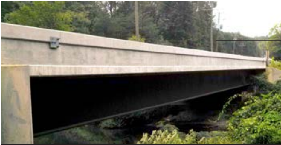
AB Consultants, Inc. Farrar Road Bridge at Davison Army Airfield (Ft. Belvoir, VA)
