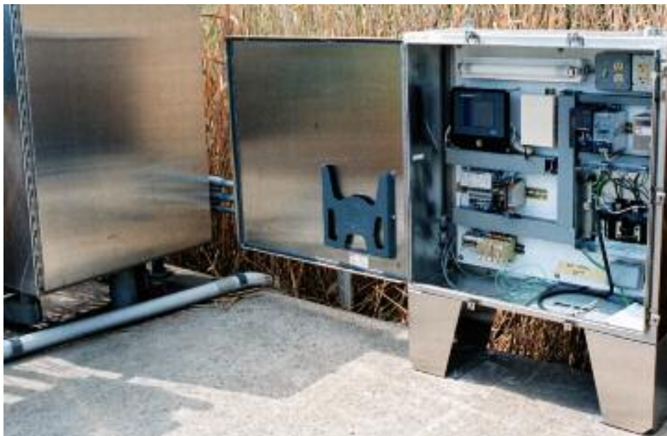
HONOR AWARD IN BUILDING/TECHNOLOGY SYSTEMS - Telemetry/Alarm Control Instrumentation for Water Distribution System - Sidhu Associates
