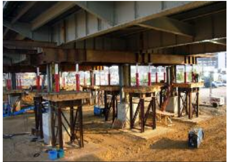
OUTSTANDING PROJECT AWARD IN TRANSPORTATION - Rehabilitation of Frederick Douglass Bridge over Anacostia River - Design/Build Project- Rummel, Klepper & Kahl
