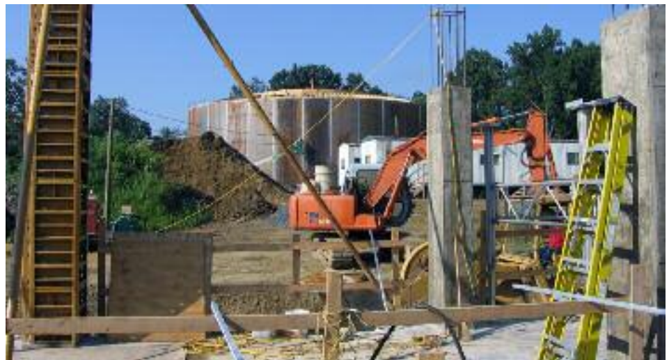
HONOR AWARD IN ENVIRONMENTAL - New Design Water Transmission System - Whitman, Requardt & Associates
